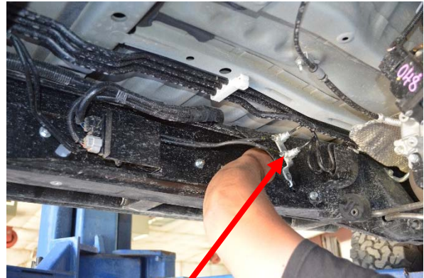
Bracket and lines moved in order to allow installers arm to fit into frame cutout
